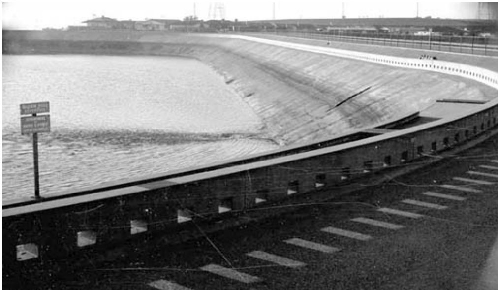
Figure 7-9: Initial Failure of Baldwin Hills Dam. Dark spot in lower right-hand quadrant shows the beginning of the break in the dam.
