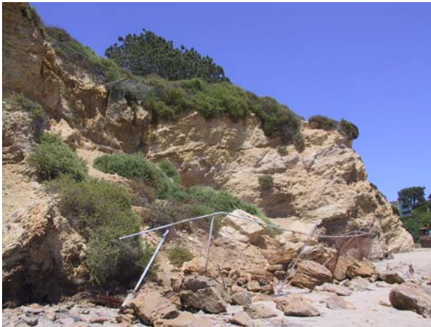
Geologic hazards such as slope failures occur in Newport Beach
