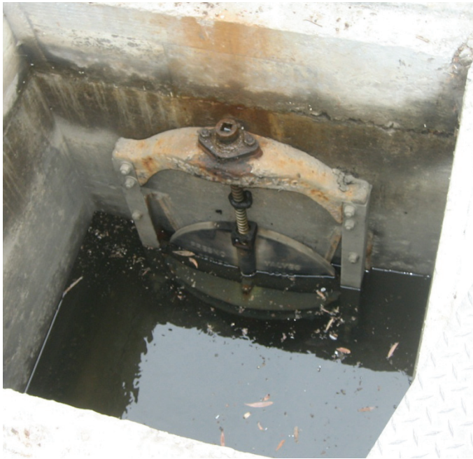
Figure 4.10 Hand-Operated Gate Valve in Storm Drain Manhole
