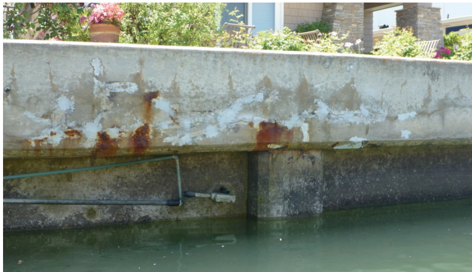
Figure 4.7 Crack Repairs with Corroding Rebar
