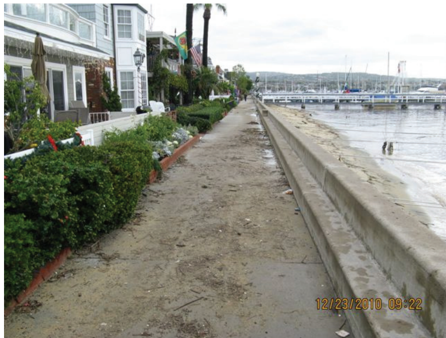
Figure 1.7 Accumulated Sand and Debris, Post-Storm
