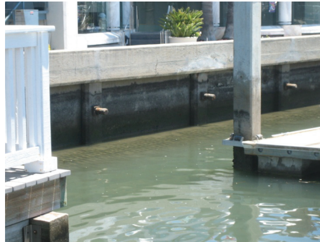
Figure 4.2 Earth Anchors and Concrete Block Revetment (Submerged) at Balboa Island Ferry Boat Landing
