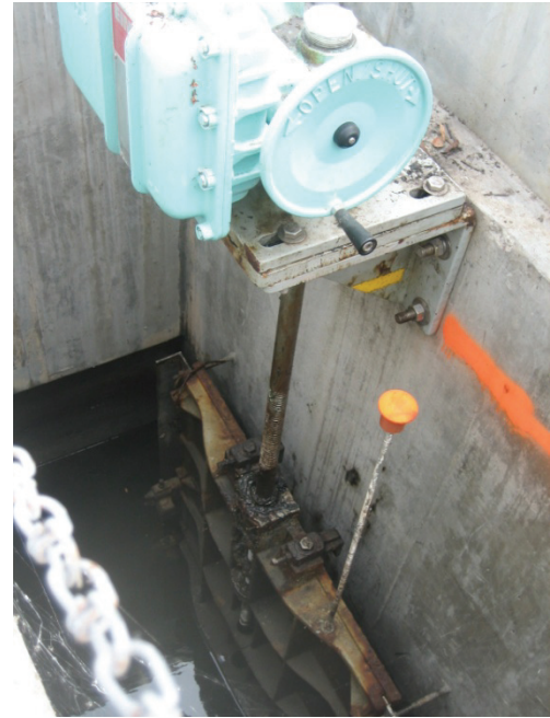
Figure 4.11 Actuated Gate Valve in Storm Drain Vault
