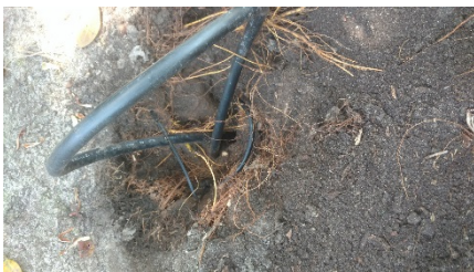
Before - Old copper cable sticking out of the ground and the hand hole where the conduit should be, is completely covered.
