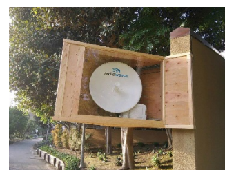
The Antenna had to be mounted low on the building to go below the trees in order to connect to OASIS Senior Center.
