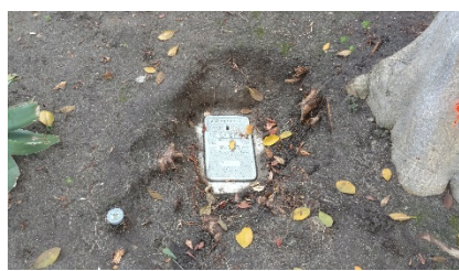
After - Tree roots have been cut and dirt was cleared out to reveal the hand hole so AT&T could bring fiber into the building.
