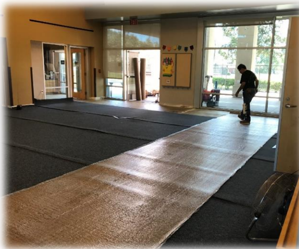
Carpet replacement in the Mariners Vincent Jorgensen Community Room at Mariners Park
