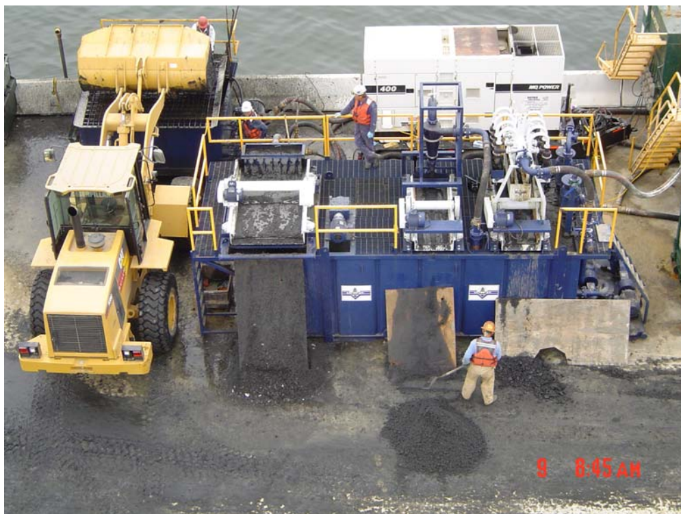
Figure C-5 Aerial view of Tri-Flo International Hydrocyclone and Scalper Unit
