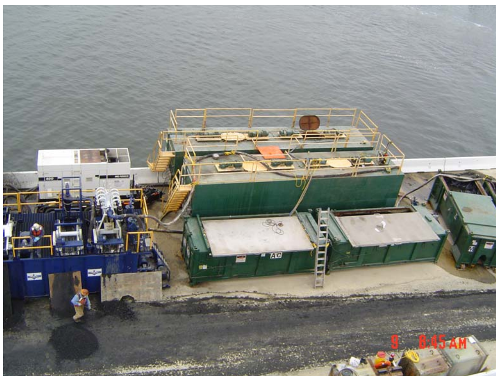
Figure C-6 Aerial View of Hydrocyclone, Baker Tanks, Settling Tanks and Generator
