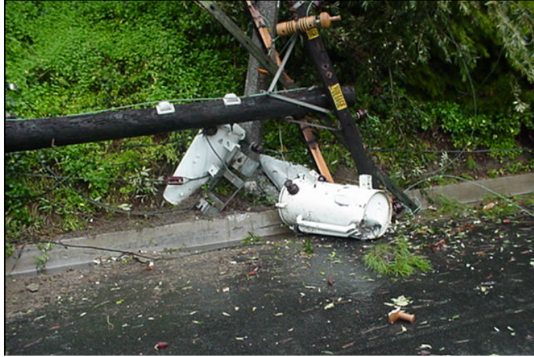
Figure 10-5: Downed power lines (and transformer) in the City of Newport Beach caused by the January 1, 2005 storm.
