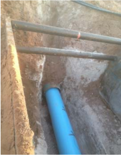
Exposed Water Main
