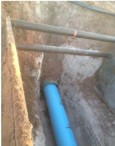
Exposed Water Main
