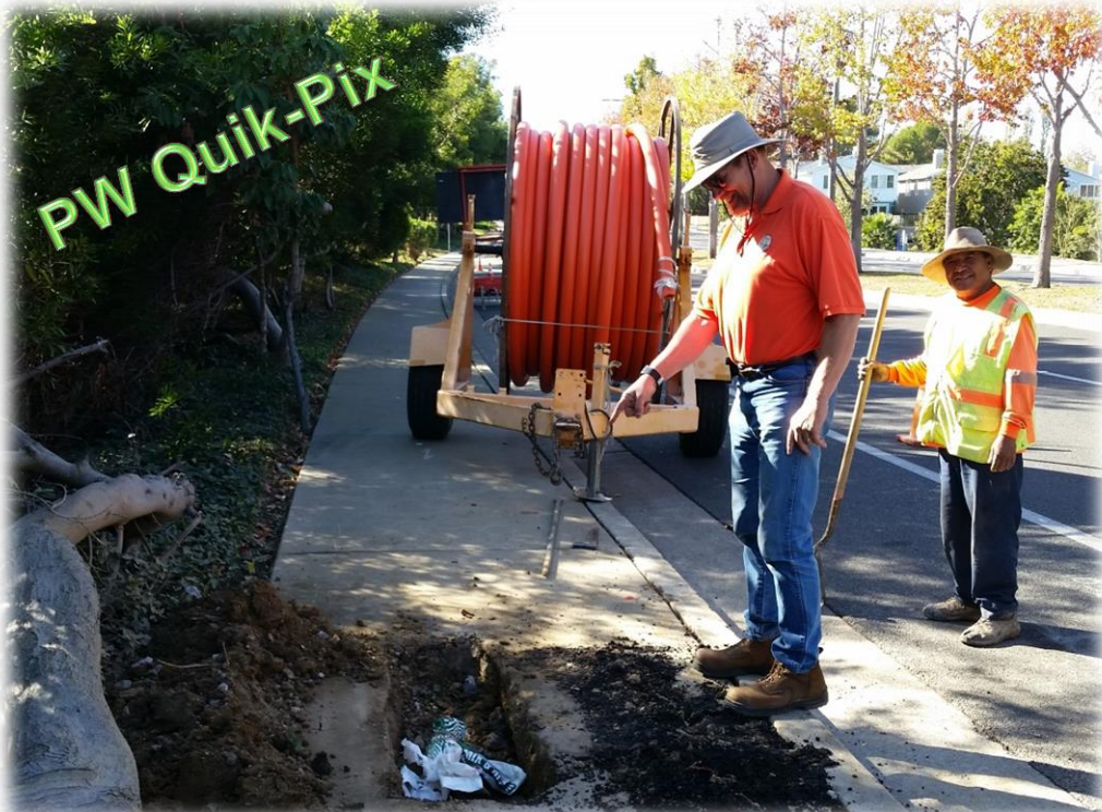
Senior Inspector Mike St. Clair examines the fiber optic conduit for the Signal Modernization Project on San Miguel
