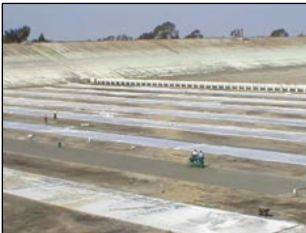
During this fiscal year, Big Canyon Reservoir, located in Corona Del Mar, will be covered and a new treatment facility will be added. The covering of the reservoir will help to improve water quality. In this picture, workers are making necessary repairs to the bottom of the empty reservoir. Once the surface repairs are complete, the installation of the floating cover will begin.
