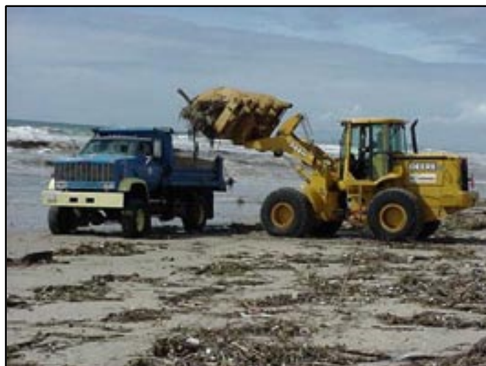
Beach Maintenance following a winter storm
