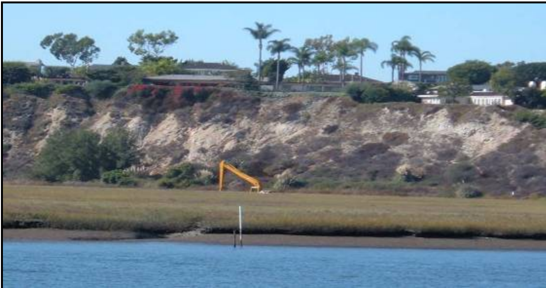
Amphibious Excavator working in Middle Island Channel, photo by Jay Grandon, October 2008
