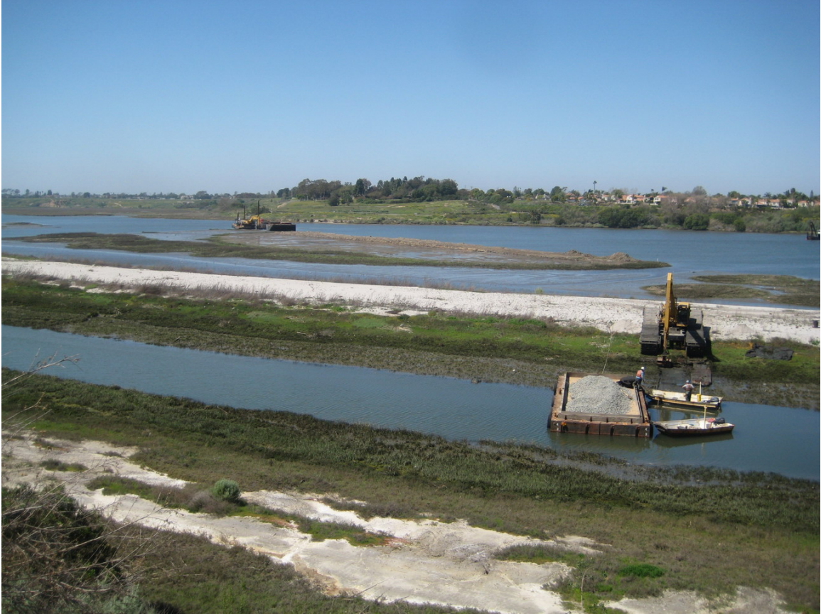
Hotdog Tern Island Ramp Construction, Removal of Skimmer Island and Unit I/III Sediment Basin Dredging, March 2010, Photo by Greg Fuderer
