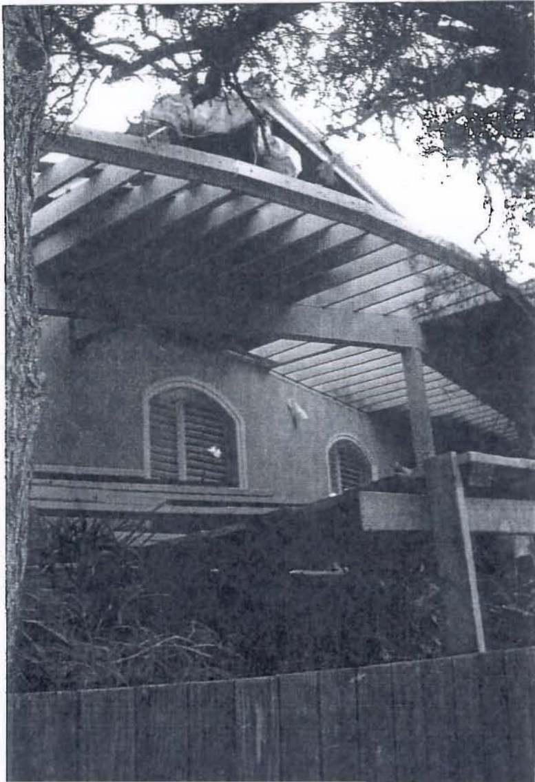
436 Riviera Terrace (directly across the street from 444 Mendoza) (planks on deck are currently being replaced)
