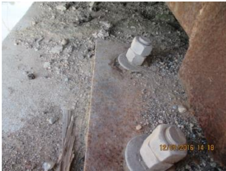
The anchor bolts are no longer vertical and bent away from the creek at South Abutment
